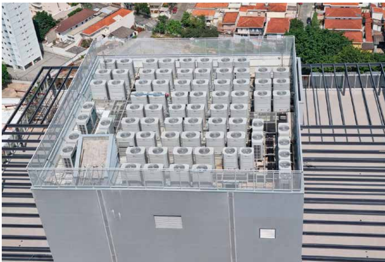
Cobertura com as condensadoras VRF
